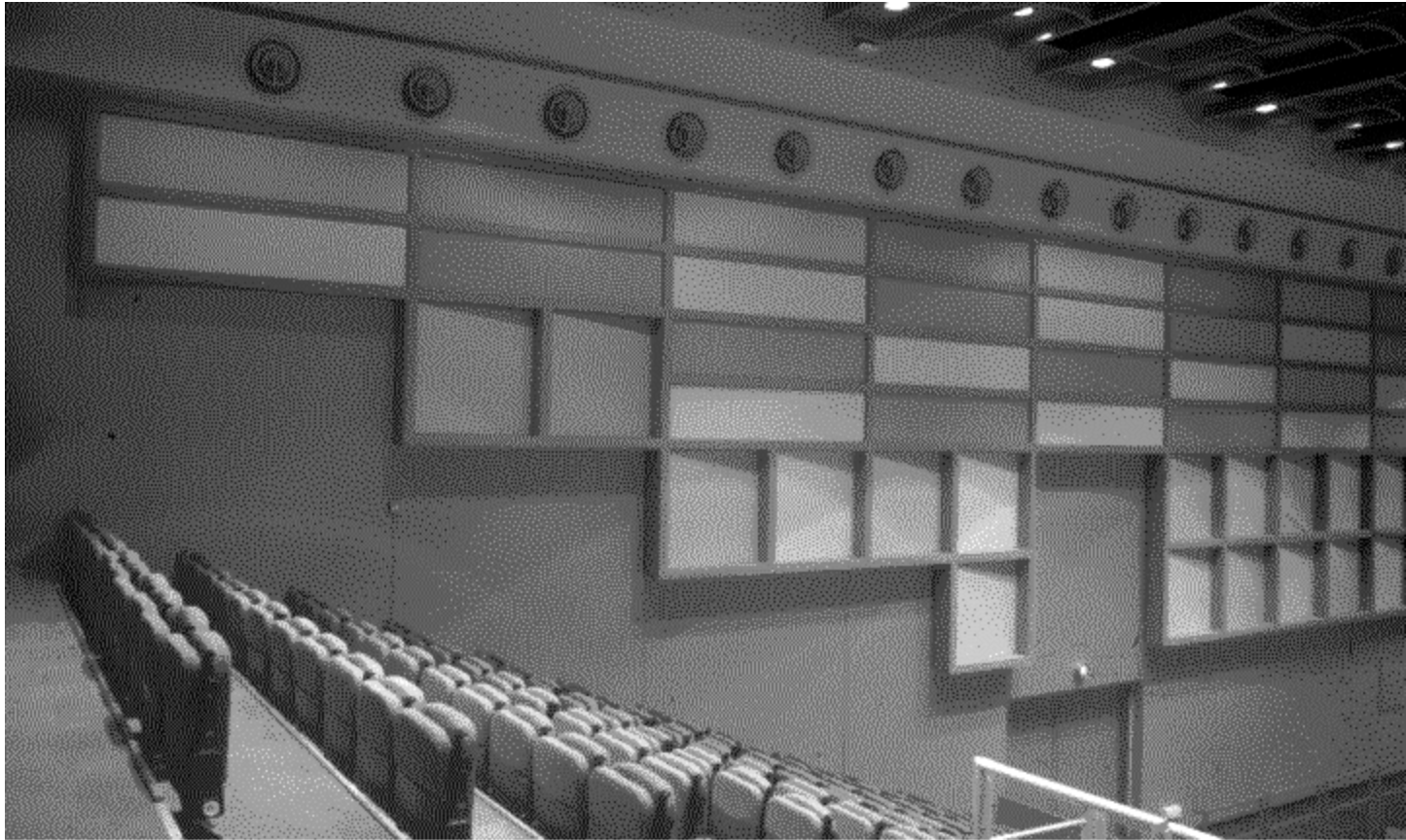
Fig. 4.3.6 Example of membrane absorbers attached to the concrete side wall in the multi purpose hall (Kolding Teater). Besides controlling low frequency reverberation, the panels also provide some diffusion of the sound.
